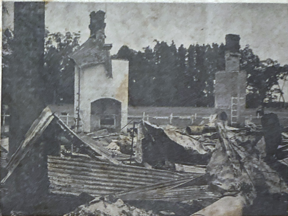
● ● The remains of the old Forests Department's Ludlow school building lie smouldering after last Saturday morning's blaze.
